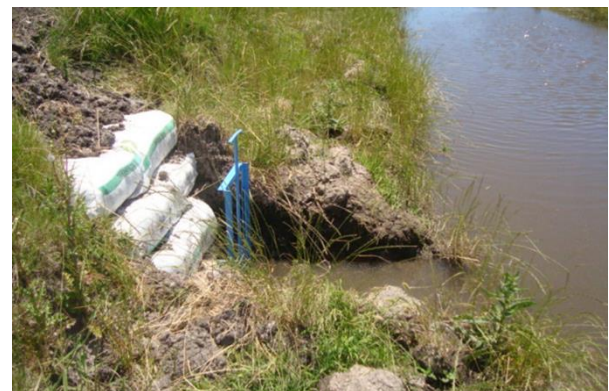
Figure 1. Pipe gate installed at the entrance of a production plot
